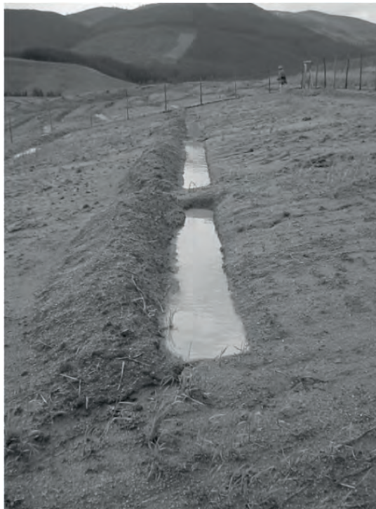
Figure 2.7. A contour trench constructed a hillslope to reduce the velocity of surface runoff, impound runoff water, and decrease surface erosion by retaining runoff water and entrained soil particles (photograph by Roberto Pizarro Tapia).
