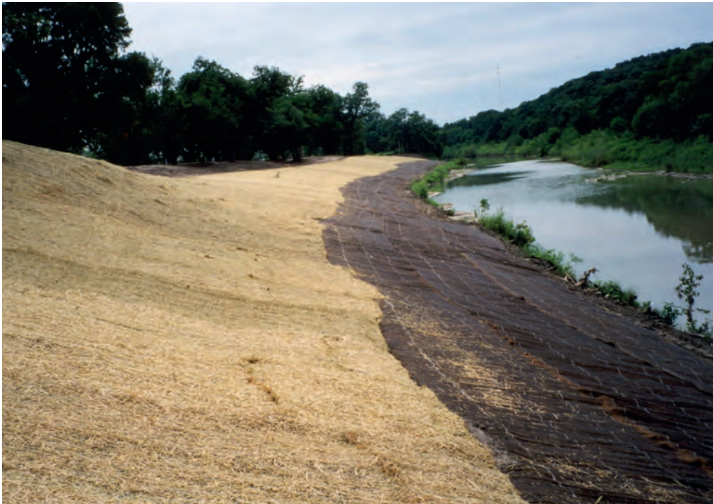
Figure 2.4. An erosion-control blanket placed on an eroding hillslope to facilitate establishing a vegetative cover by protecting the soil surface from the impacts of rainfall events and surface runoff (image from North American Green at www.nagreen.com ).
