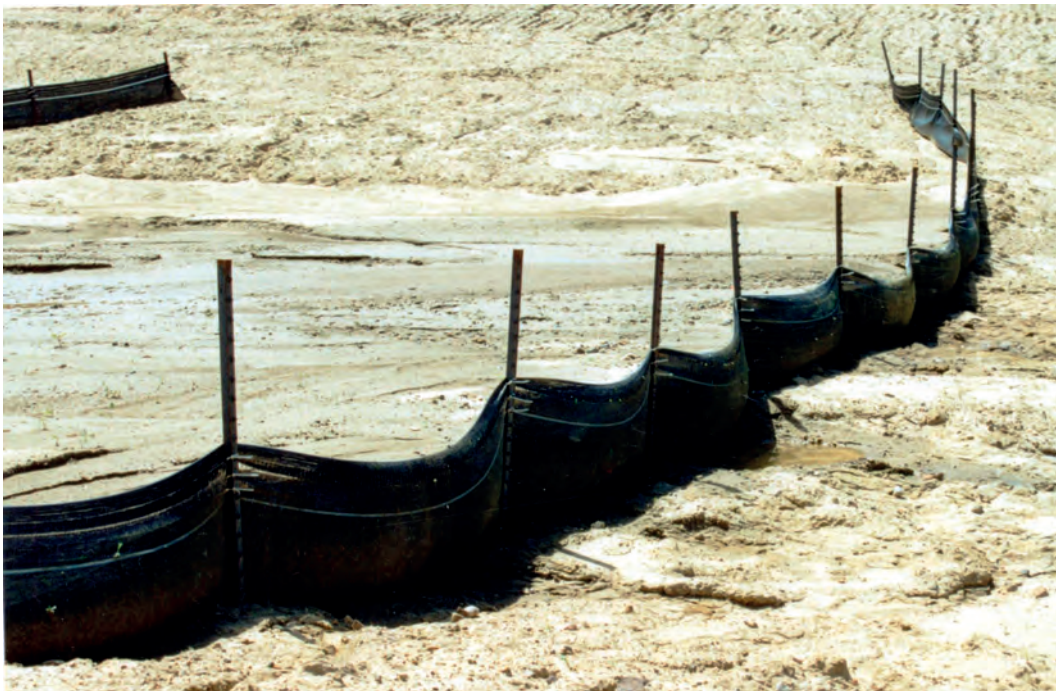
Figure 2.5. A silt fence installed to temporarily control surface erosion on a hillslope. Soil particles entrained in surface runoff are captured on the uphill side of the fence through the settling of water (image from Thomas Carpenter, CPESC).
