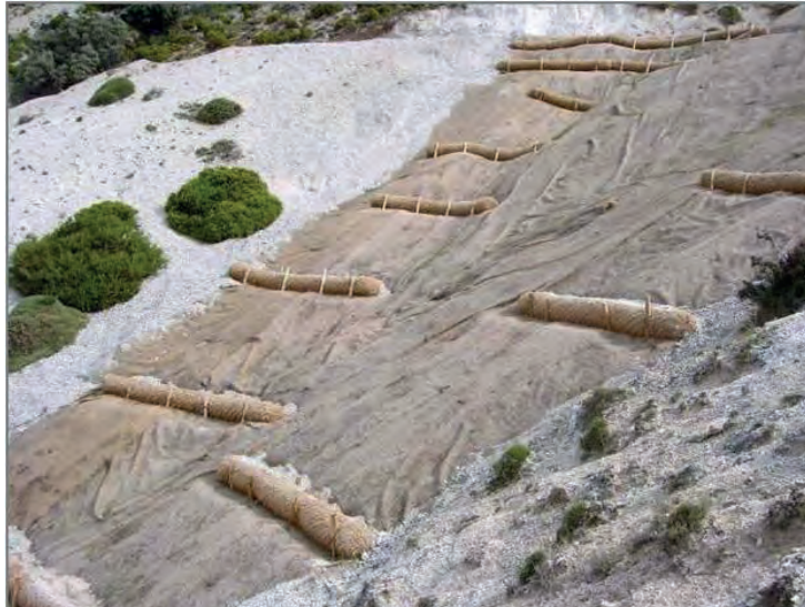
Figure 2.6. Straw wattles placed along the contours of an eroding hillslope to stabilize the slope and control surface erosion (image from BonTerra Iberica at www.bonterrailberica.com ).
